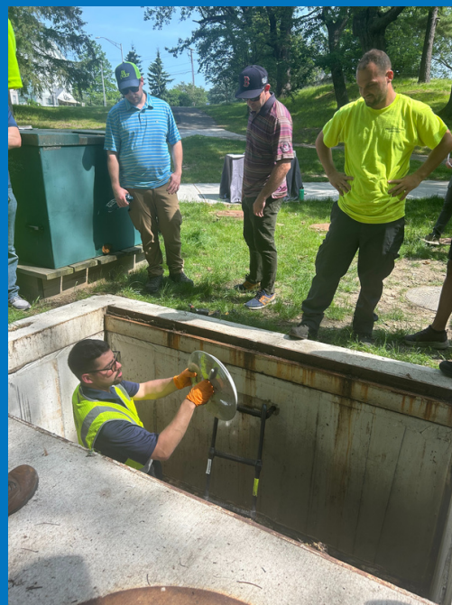
LidTech/Stormwater Compliance COO Nate Marles demonstrating how to clean the jellyfish filter
