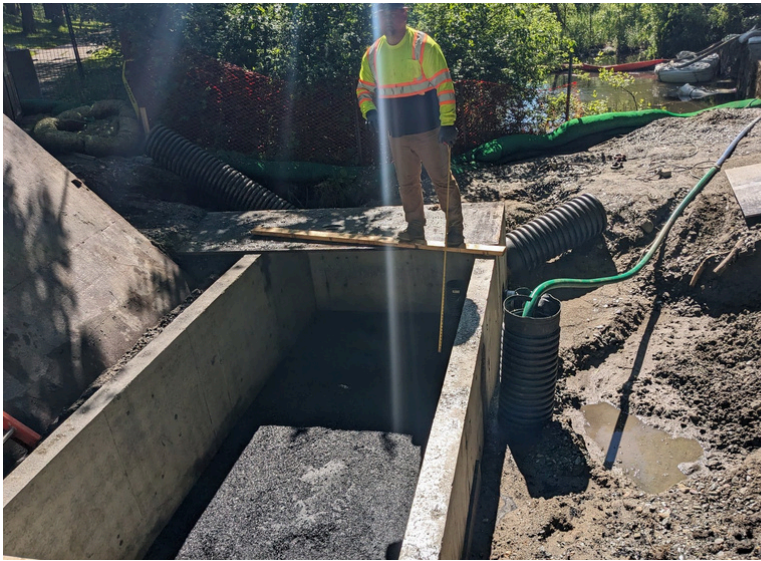
Treatment Train vault filled with biochar
